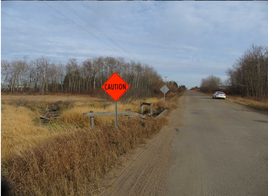
6. Caution signs warning of missing bridge rail
