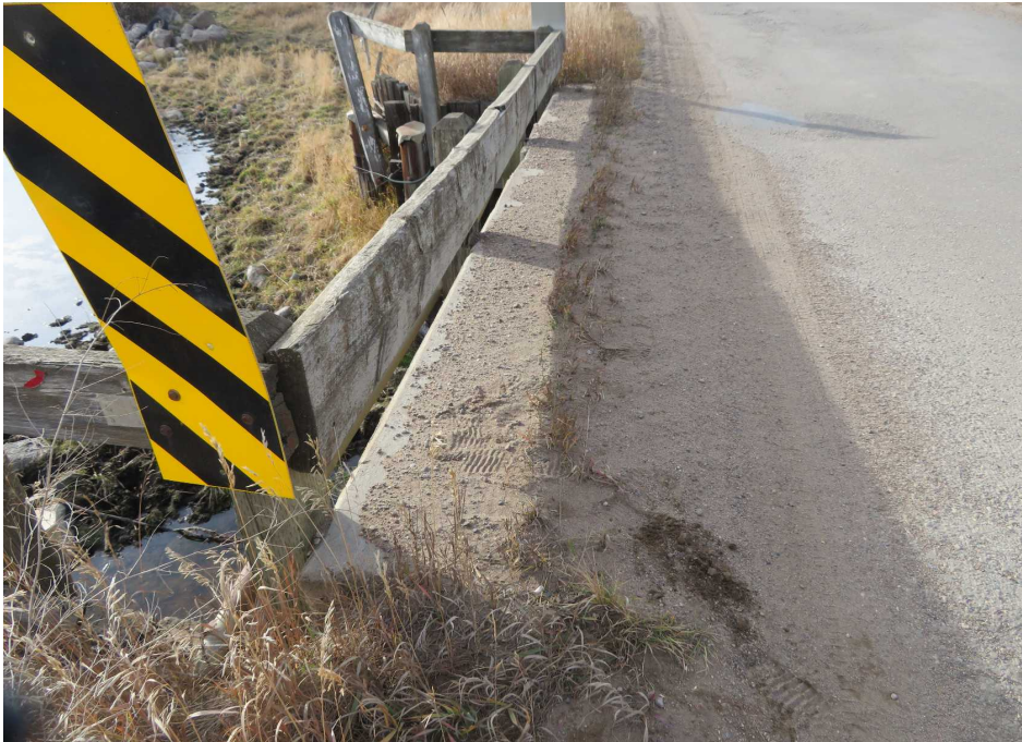
7. Silt along south curb. Cold mix to top of curbs
