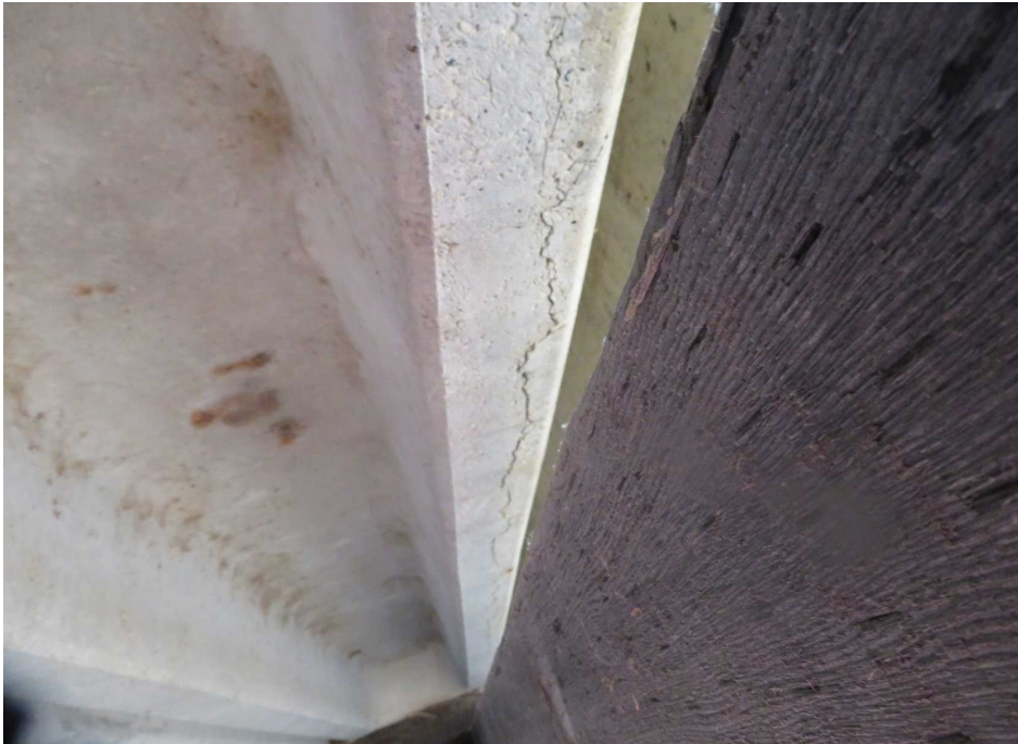
13. G3- medium crack in 1 leg
