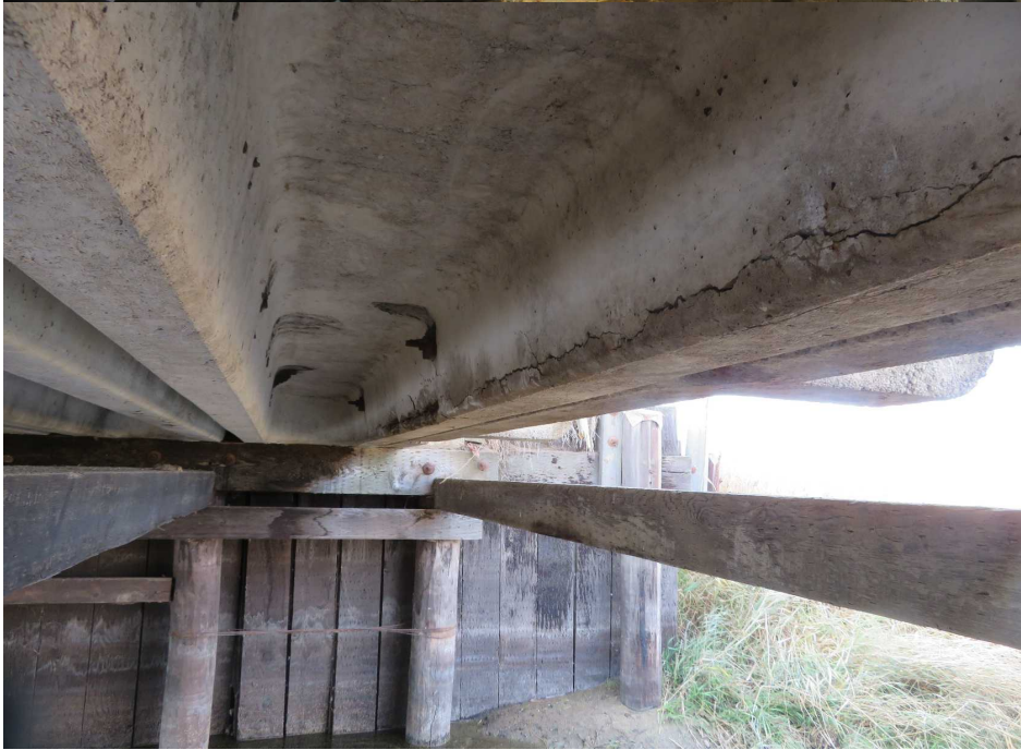
12. G8- spall in 1 leg out of AZ. Wide crack in both legs.
