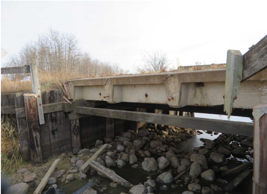
5. Profile. Note missing north bridge rail
