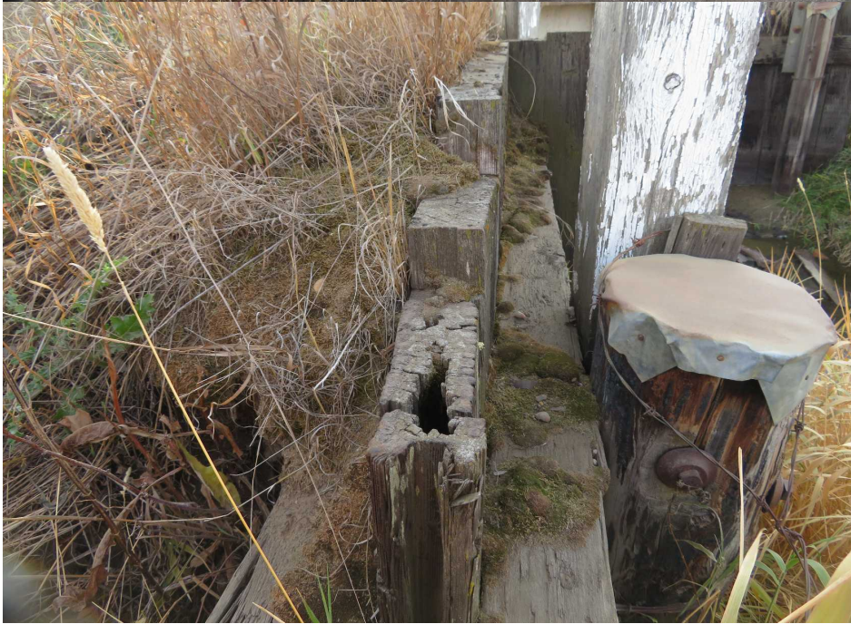
8. N/E wing vertical planks rotten
