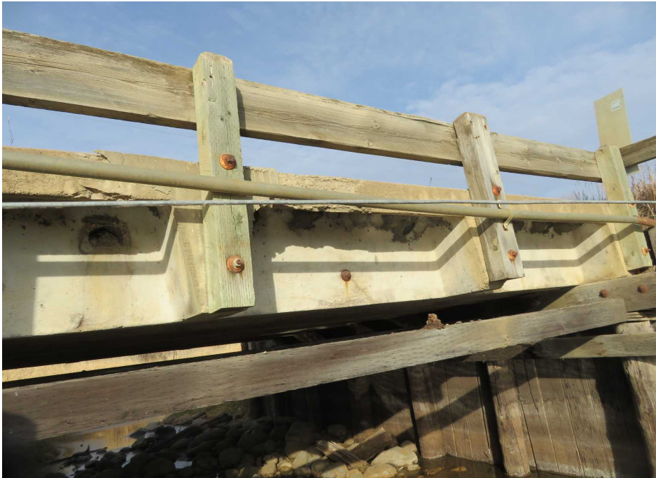
11. South curb unit-spalling
