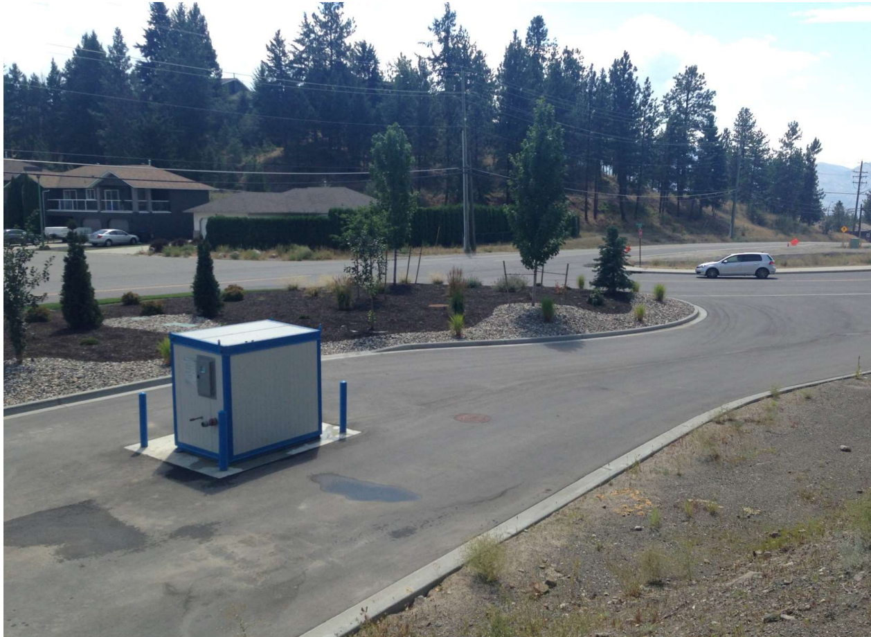
Marwayne Reservoir Bulk Water Fill Station
