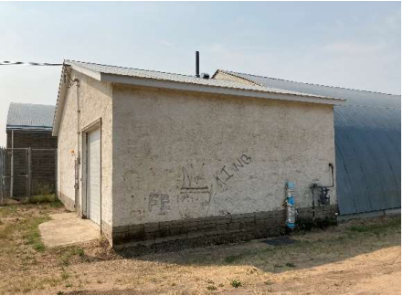
Picture #9.4 – Mechanical Room.
