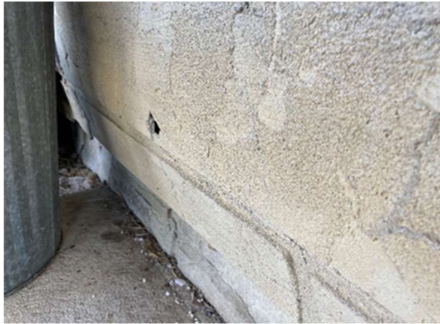
Picture #6.4 – Bulging of the Foundation Wall at the Top.
