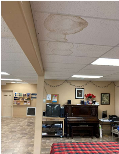
Picture #5.6 – Water Staining on the Ceiling Tiles.
