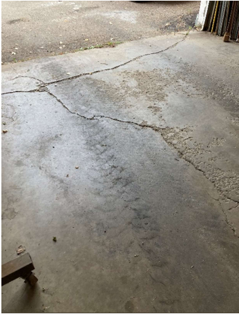
Picture #3.3 – Cracks and Wear on Concrete Shop Floor.
