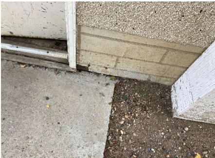
Picture #3.5 – Hole in Exterior Wall Finish of the Shop. Deterioration of the Wood Framing for the Door was noted.
