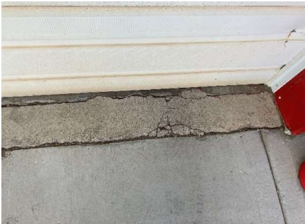
Picture #4.6 – Cracking at transition between interior slab and exterior apron slabs.
