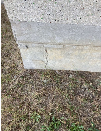
Picture #6.3 – Vertical Cracks in the Foundation.
