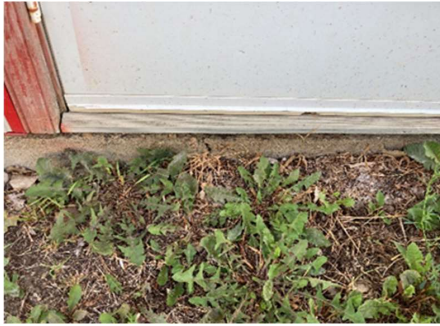
Picture #4.9 – Deteriorated Door Trim, and Weather Stripping.
