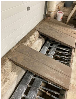
Picture #8.11 – Spalling Concrete on the East Side of the Arena.
