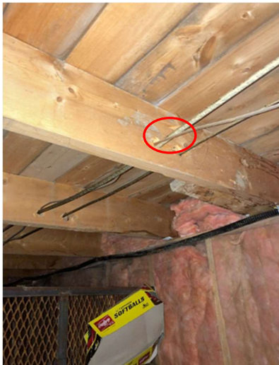
Picture #6.5 – Crack in Floor Joist, Partially Obstructed by Wires.
