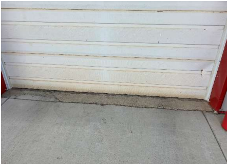
Picture #4.8 – Damage to Exterior Overhead Door.
