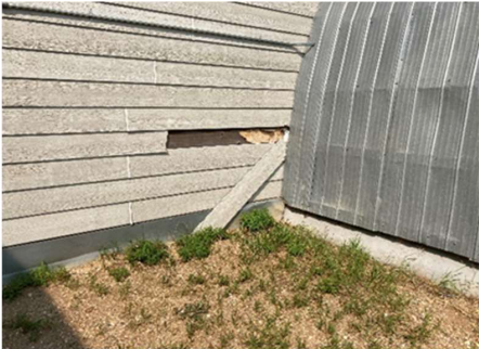
Picture #9.5 – Missing Siding Board.
