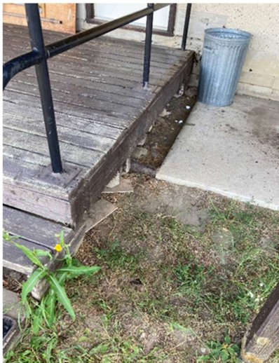
Picture #6.15 –Canopy Steps and Deck Supported by Combination of Concrete Blocks and Directly on the Ground.
