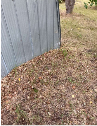
Picture #7.3 – Debris Piled Next the Quonset.
