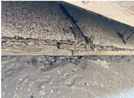
Picture #9.11 – Metal Cladding Separating from the Shingles.
