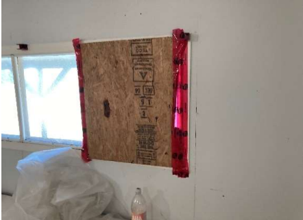
Picture #6.8– Missing Window.
