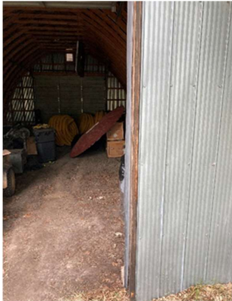
Picture #7.7 - Deteriorated Trim Around the Overhead Door.
