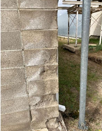
Picture #8.13 – Weathered Exterior Blocks.
