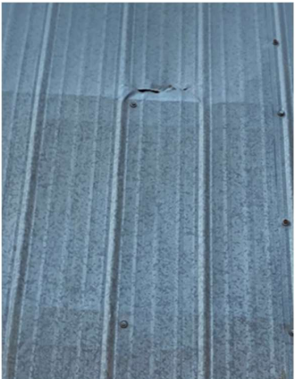
Picture #9.9 – Hole in the metal siding.
