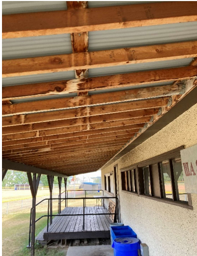
Picture #6.13 – Deteriorated Canopy Framing.
