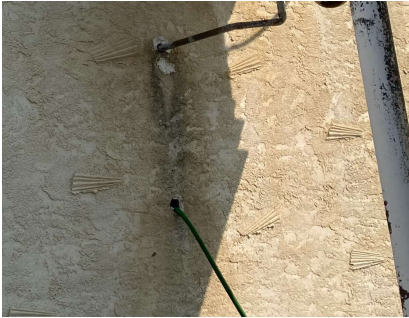
Picture #9.13 – Poorly Sealed Wall Penetrations.
