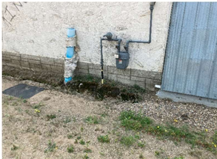
Picture #9.12 – Deteriorated Exterior Finishes of North Side of Mechanical Room.
