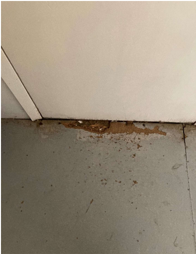
Picture #6.5 – Worn Floor Finishes.
