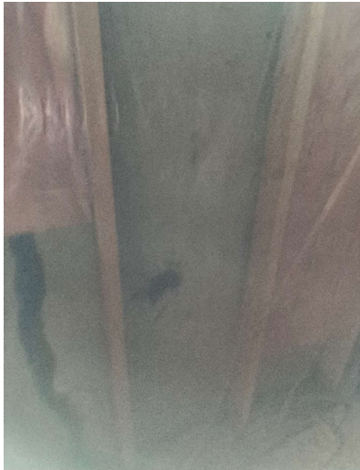
Picture #6.10– Missing Insulation and Wall Finishes in the Basement.
