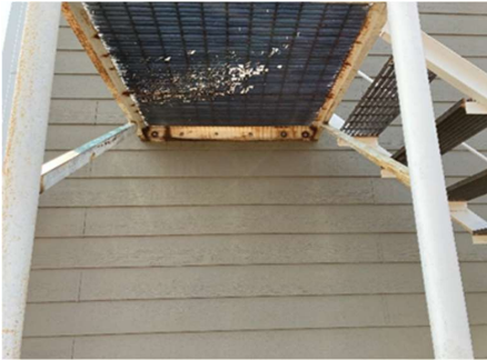
Picture #9.7 – Rusted Exterior Stairs.
