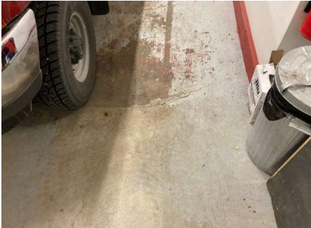
Picture #4.5 – Crack and Wear on Concrete Garage Floor.
