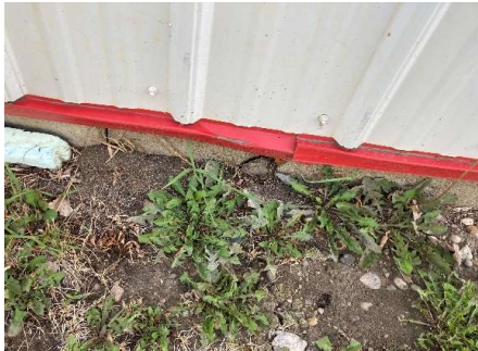
Picture #4.3 – Cracks in West Foundation.
