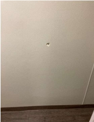
Picture #8.6 – Hole in Interior Drywall.
