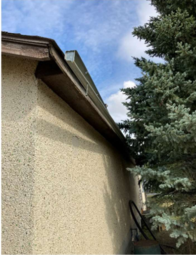
Picture #6.12 – Trim and Downspouts Separating for the Roof.
