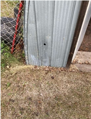
Picture #7.5 - Hole in Metal Siding of the Quonset.
