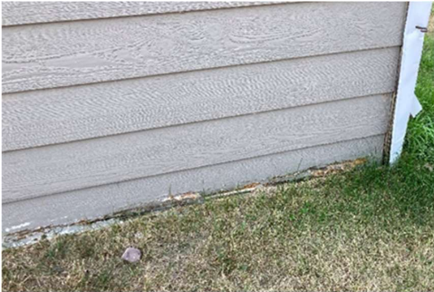
Picture #9.6 – Deterioration of siding around the base of the lobby's exterior wall.
