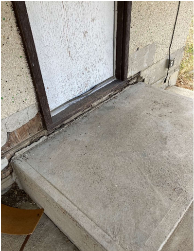
Picture #6.7– Failed Exterior Wall Finishes with Rotting Wood Behind.
