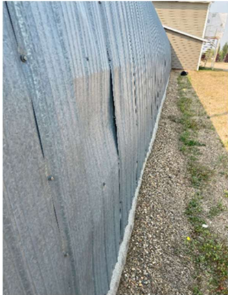
Picture #9.10 – Gap in the Metal Siding.
