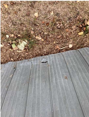
Picture #7.6 - Hole in Metal Siding of the Quonset.
