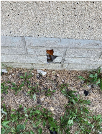
Picture #3.4 – Hole in Exterior Wall Finish of the Shop.
