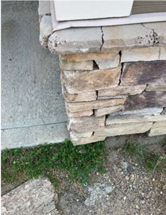
Picture #8.5 – Cracks in the Lobby Exterior Stone Trim.
