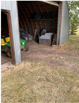
Picture #7.3a – Ground Sloping Towards the Inside of the Quonset.
