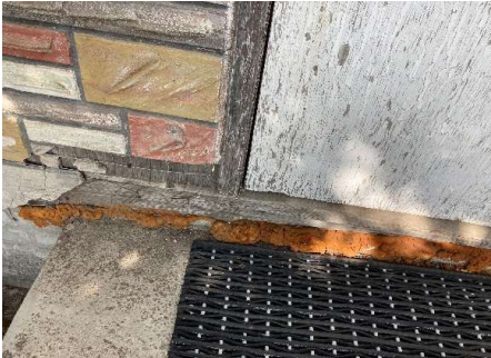
Picture #6.6– Failed Exterior Wall Finishes with Rotting Wood Behind.
