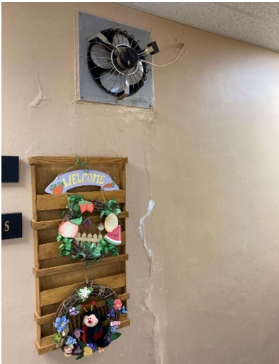
Picture #5.4 – Exhaust Fan and Water Damaged Section of the Back Wall.
