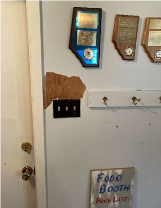
Picture #6.9– Worn Paint.
