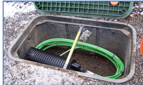
Figure 14. A typical handhole.
