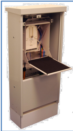
Figure 15. Fibre-optic splice cabinet.
