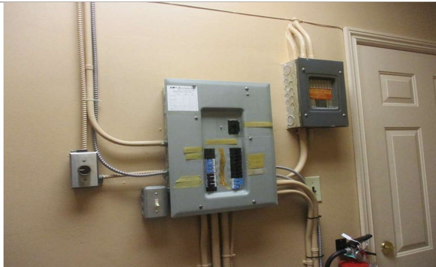
Picture location: Electrical service
