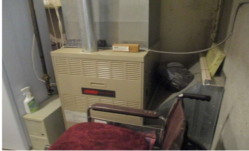
Picture location: Typical forced air furnace
